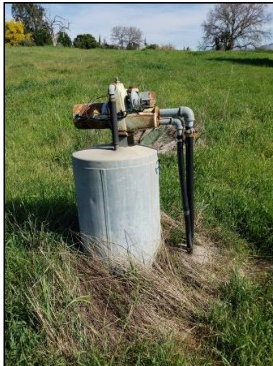
10 : View from northern parcel. Photograph depicts water well. At least one faucet was located at the tool shed.
