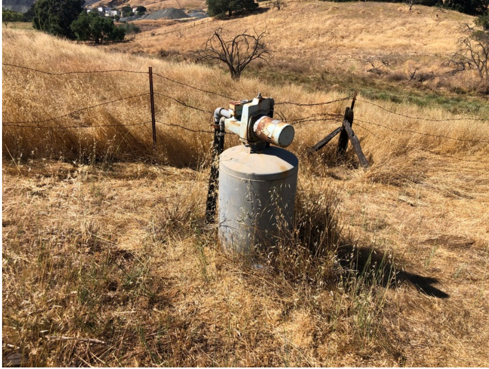
9. View of water pump on subject property
